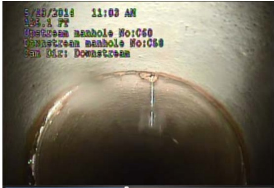
Figure 5. Gravity Sewer Line with Constant Drip from Infiltration
